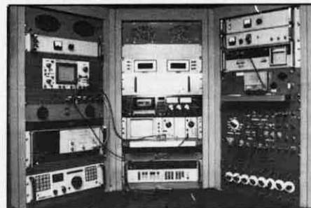
Measurement and recording racks.
